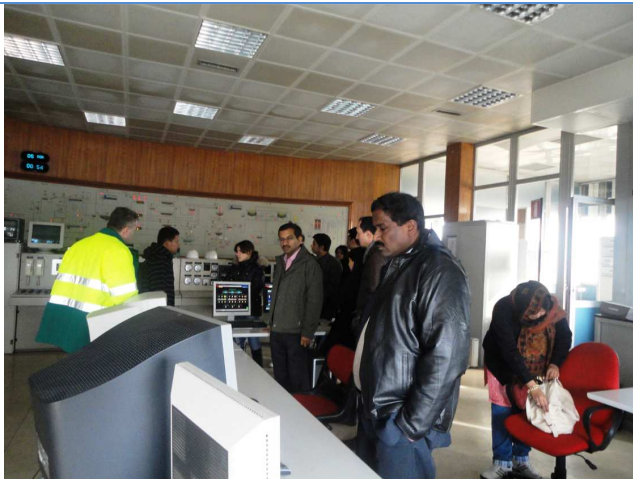
Waste Separation Plant – Control Room – Bologna.
